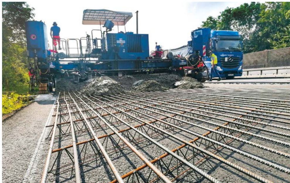
The image shows how the test stretch A61 near Boppard was built in July 2021.
