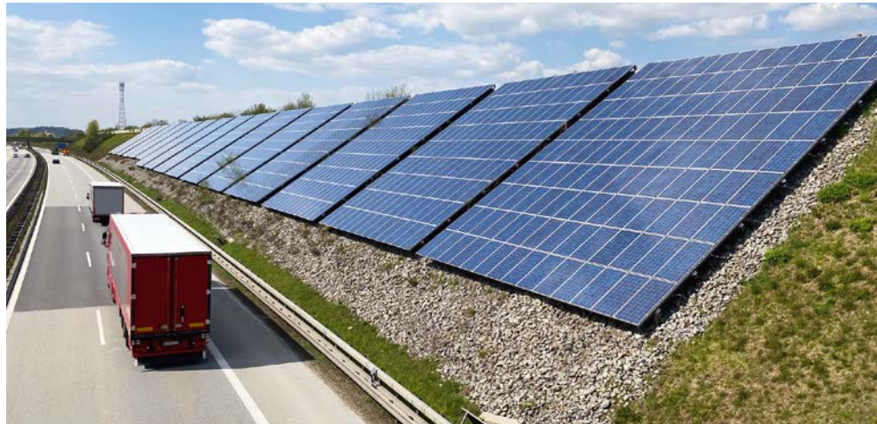
PV noise abatement wall along federal motorway A 94 near Töging.
