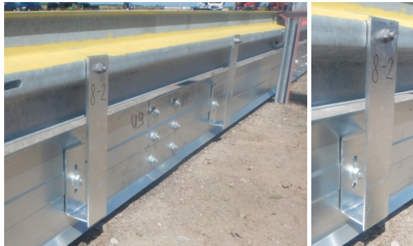
Figure 6 Mounted MPS with two-piece brackets
