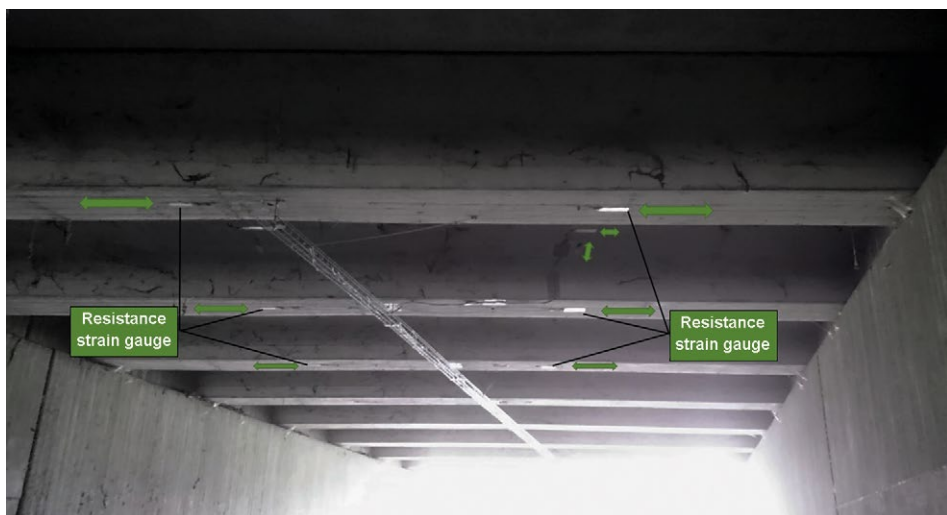
Motorway bridge with sensors to record weights of vehicles (Bridge WIM)
